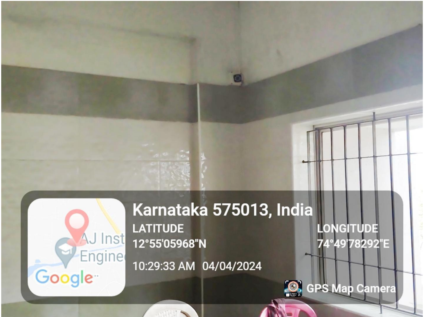
CCTV Camera Surveillance in Girls Hostel Rooms
