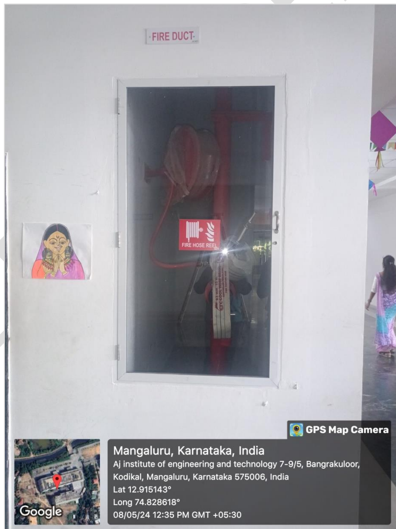
Plate 5: Fire fighting system in the premises
