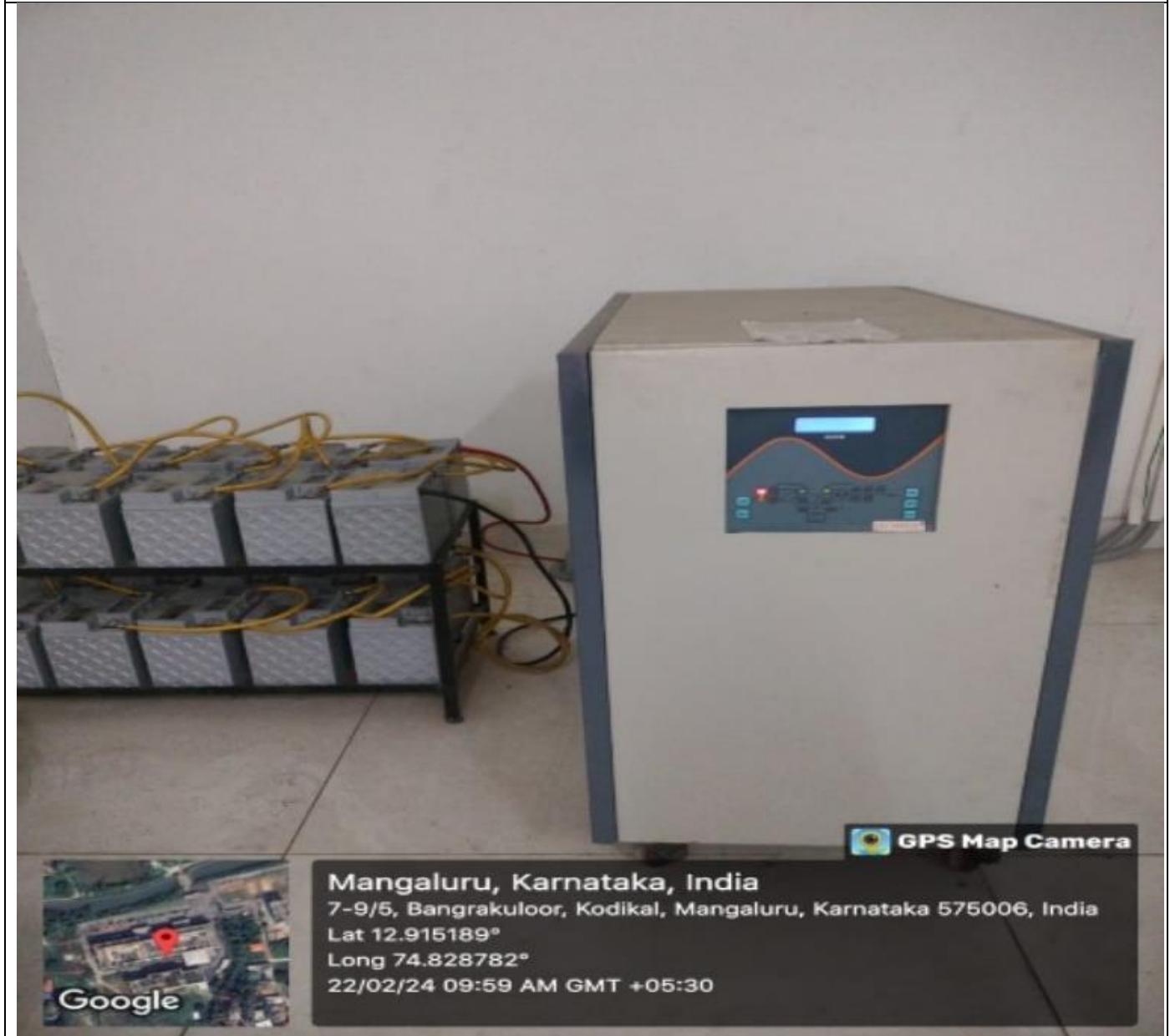
UPS FRONT VIEW
